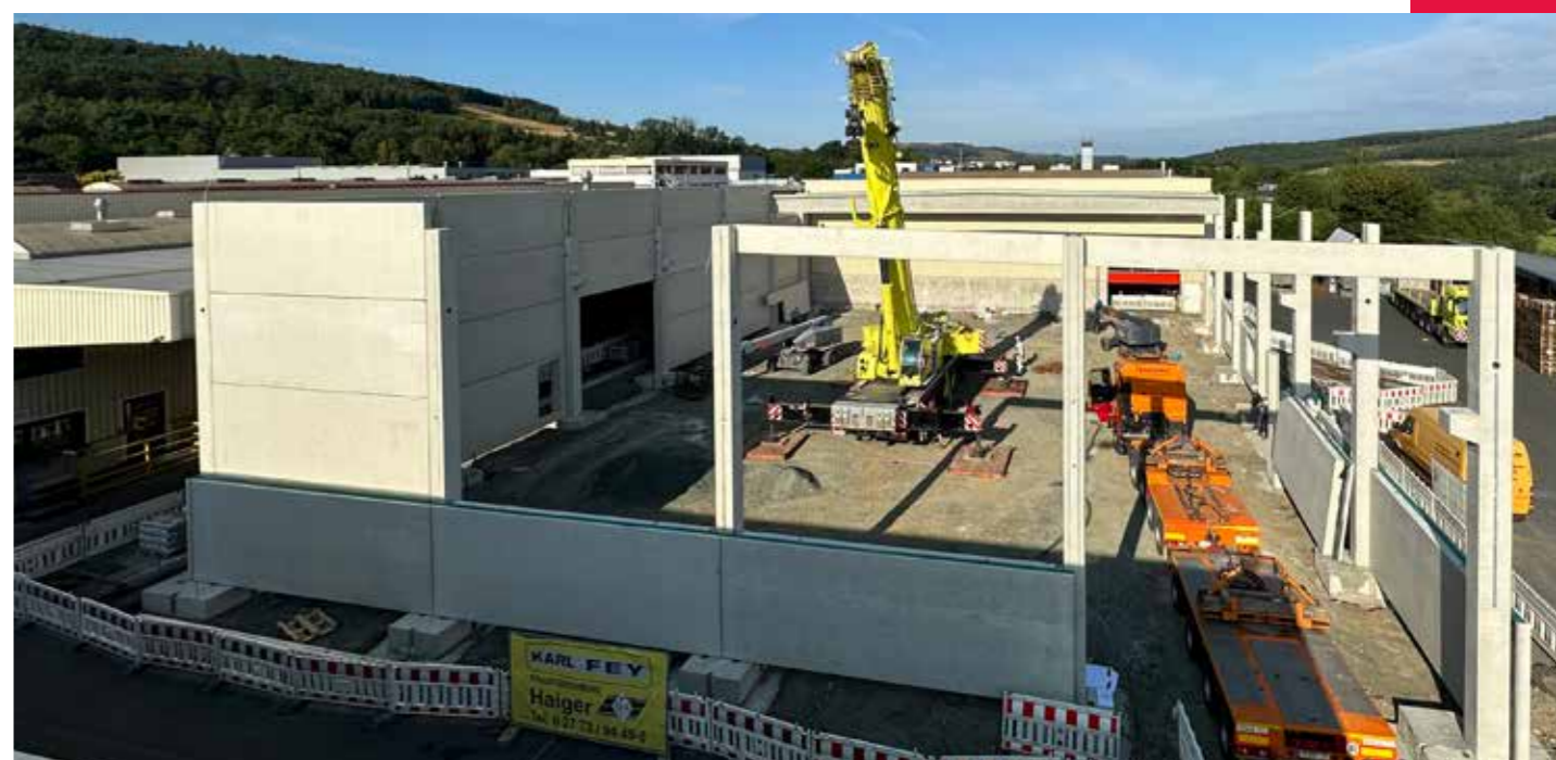
Whether conversion or site expansion, construction work never stops at VETTER, it's always going on. A lot has happened at our location in Burbach in the last year.
